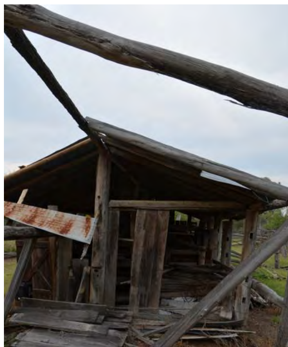
Figure 188. The north-eastern end of the milking bails structure, which is substantially deteriorated.
