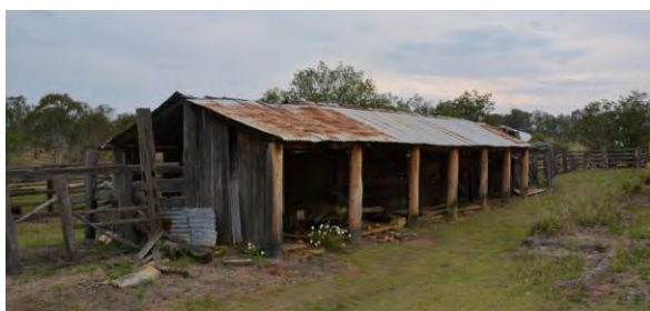
Figure 181. The north-west elevation of the milk bails structure. Note the rough-sawn timber slabs, fitted vertically, that partially enclose the structure at this end and the timber posts supporting the structure.
