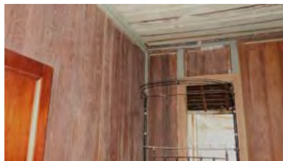
Figure 113. The south-east corner of Bedroom 2, which is showing evidence of water penetration affecting the timber ceiling fabric.
