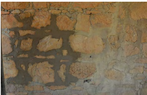
Figure 139. Detail of a section of re-pointed stonework utilising the incorrect mortar mix, as part of previous restoration works.
