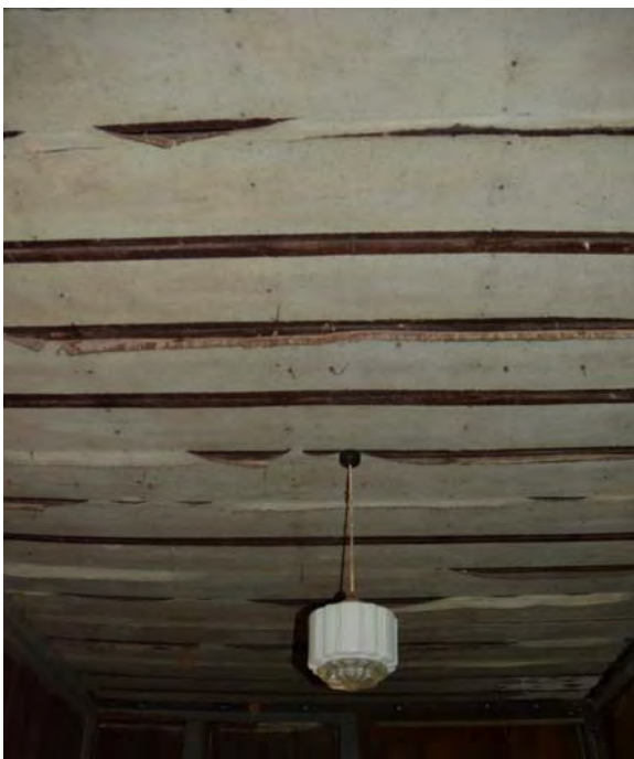
Figure 116. Detail of the dilapidated calico ceiling lining in Bedroom 2.
