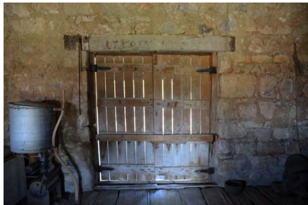
Figure 144. Detail of the timber double doors, which provide access to the stone store.
