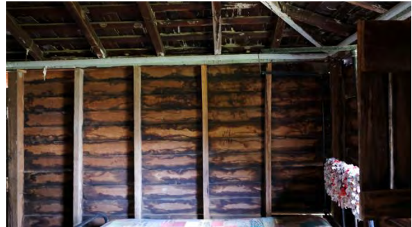
Figure 119. Interior of Bedroom 3 showing the single-skin construction framing exposed in this room.
