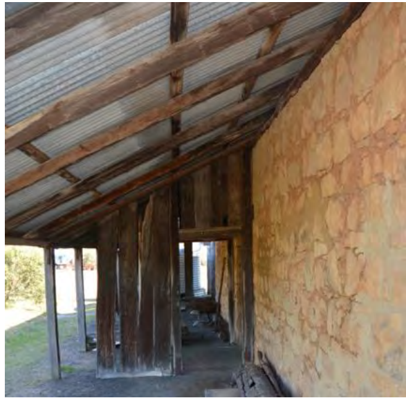
Figure 136. Example of the post-and-sapling frame construction of the lean-to verandah additions, which are reconstructions of earlier features.
