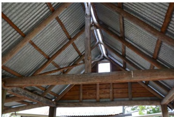
Figure 159. Interior view of the reconstructed timber roof framing built using traditional bush carpentry construction.
