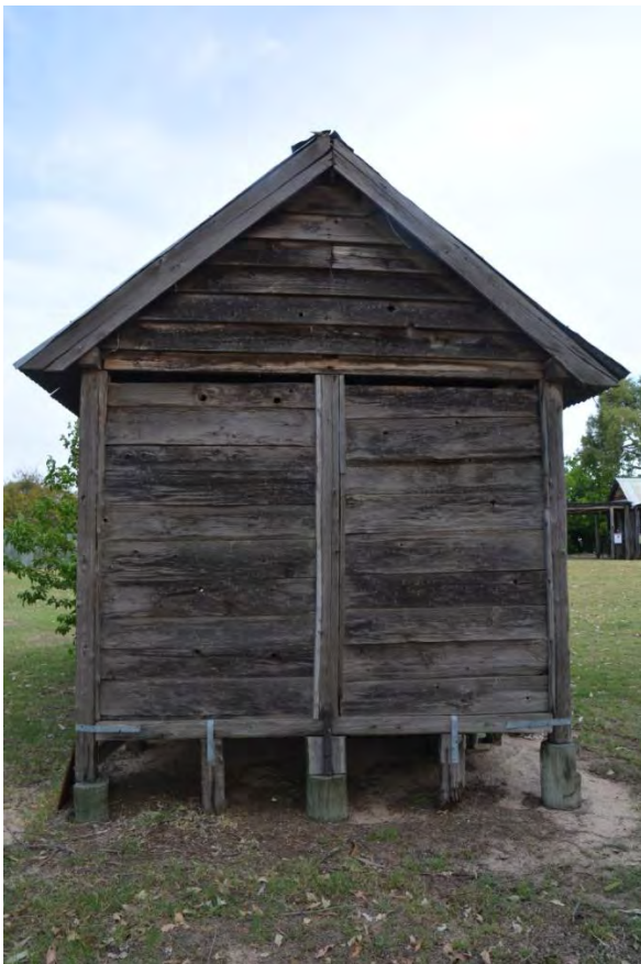
Figure 163. The rear north-west elevation of the cool house, which has been re-stumped in recent years.
