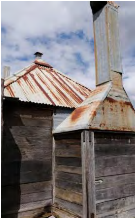
Figure 94. Rear of the detached kitchen on the south-west elevation of the main homestead, showing the pyramid roof profile and galvanised metal-clad chimney.
