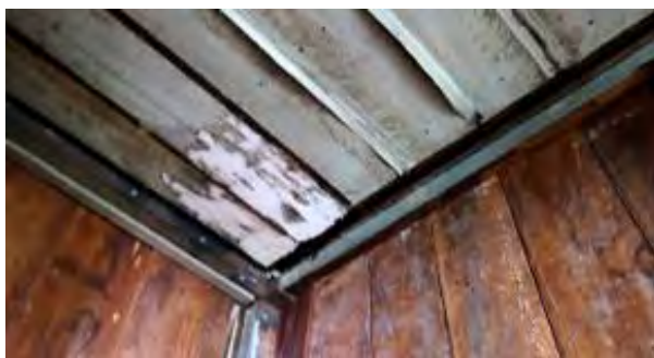
Figure 112. Detail of the north-west corner of the ceiling in Bedroom 2, showing water penetration affecting the ceiling, and movement at wall and ceiling junction.
